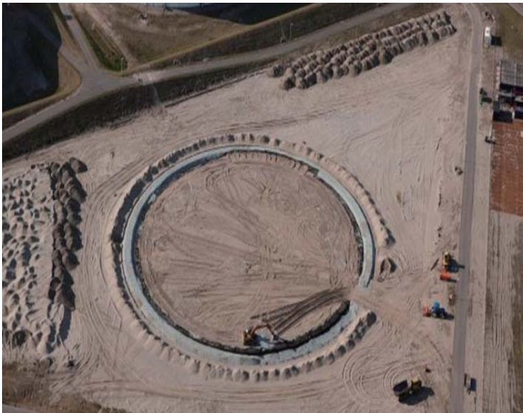
Oil Storage Tank for ATB (Malaysia)
