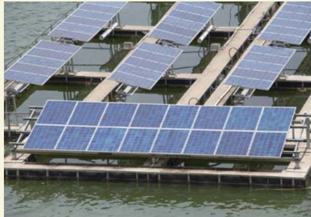
Floating Solar Power Plants
