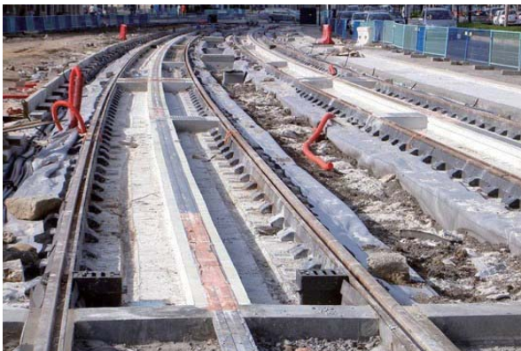
Basic Design for Construction of Honam High-Speed Railway (Korea) - Total Length : 2.9km, Station : 2ea, Underground Road : 1ea
