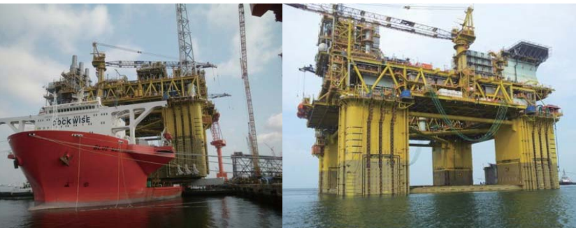
Gumusut Kakap FPSO Project (Malaysia) - Super-lift, Float-off Design and Hull FEM Analysis, Motion Analysis, Hydrodynamic Analysis, Float-Off, Transportation Detail Design and Pipeline and Flexible Riser
