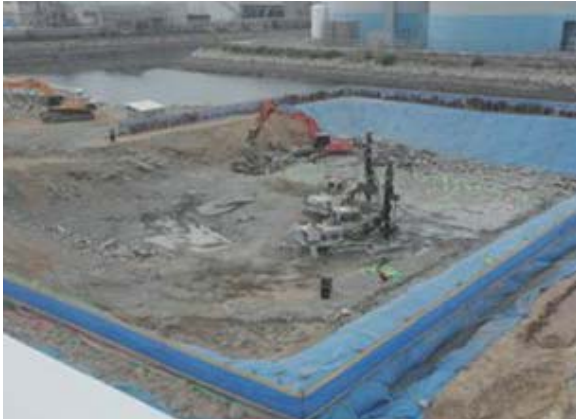
Yeosu Thermal Power Plant Project (Korea)
